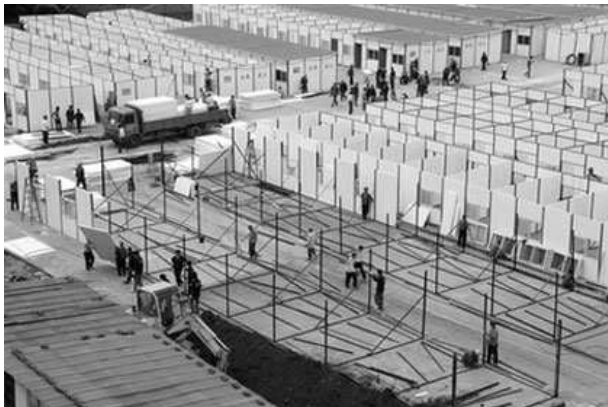
Construction workers work on a resettlement site for the victims of the May 12 quake in Dujiangyan, southwest China's Sichuan Province, May 20, 2008. A resettlement residence project has started here on May 17 and is expected to be ready on May 27. [Xinhua]
