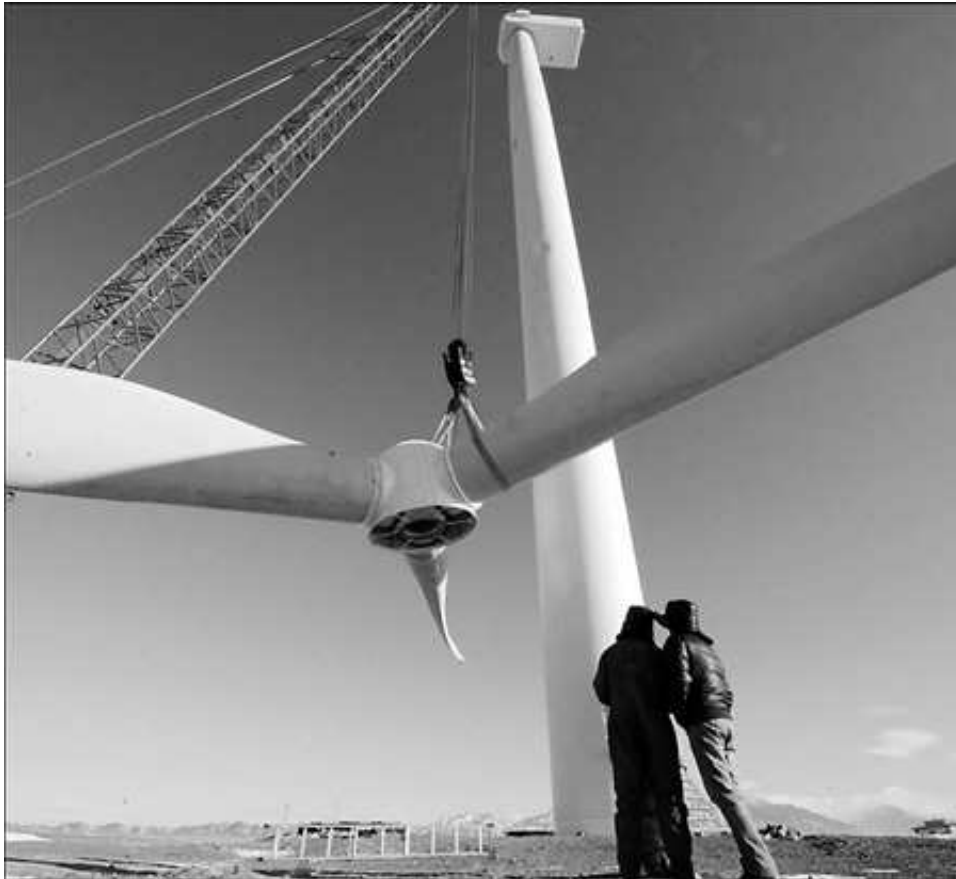
Engineers install China's most powerful inland wind turbine in Dabancheng wind field in Northwest China's Xinjiang Uygur Autonomous Region. [Xinhua]
