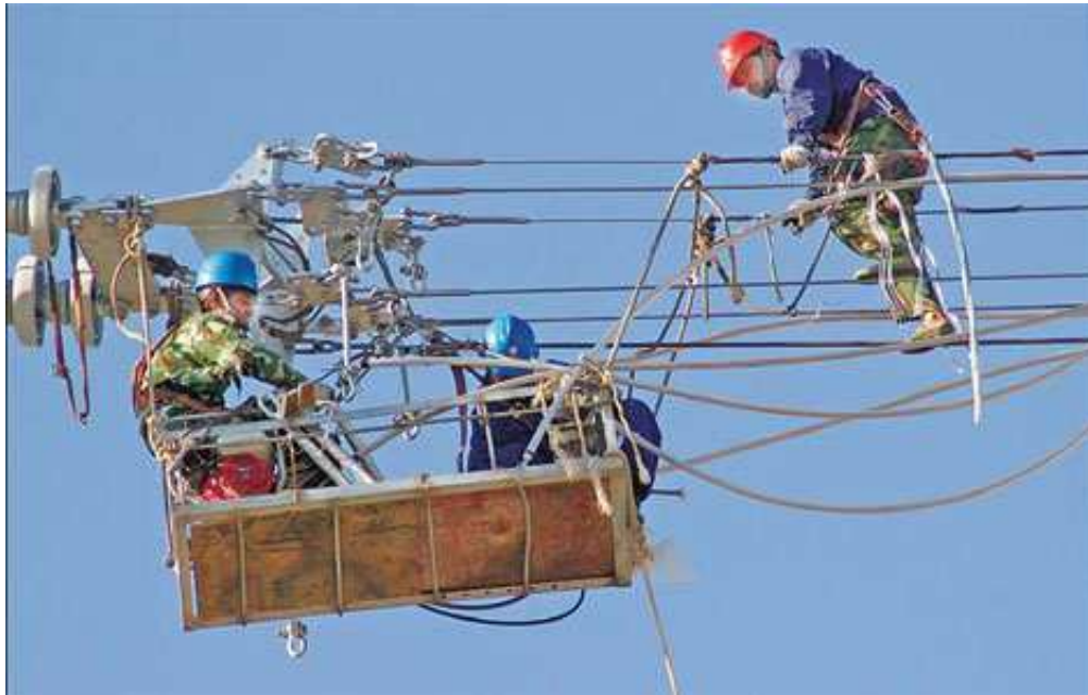
State Grid Corp workers inspect power lines in Henan province. [Cai Zengle / For China Daily]
